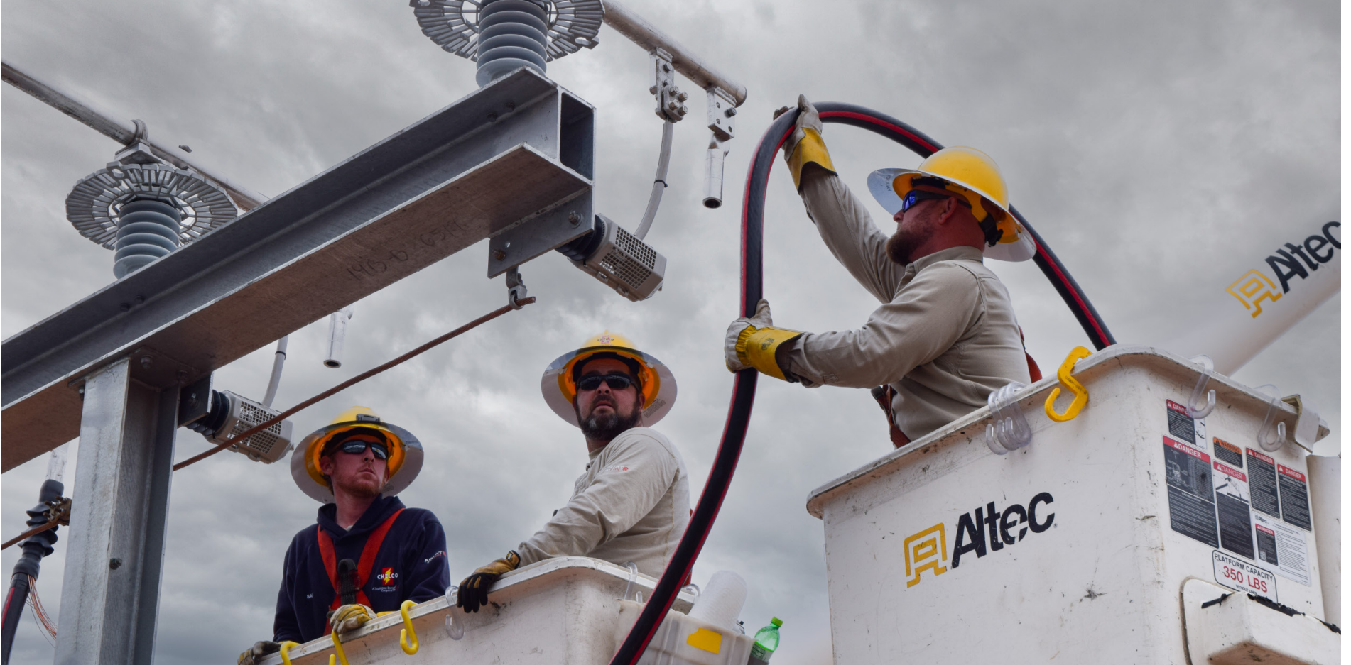
L-R: SAM DUNN, JONATHAN REED AND KALE GOMILLION MAKING INSTALLATIONS IN THE NEW OWLS HEAD SUBSTATION
